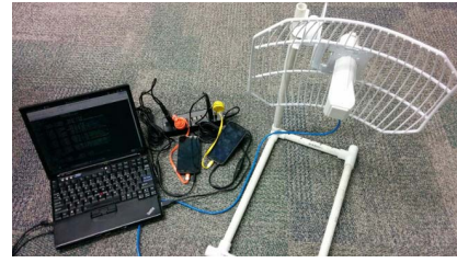
Fig. 6: PhoneHome remote node equipment. The remote node includes a PC, GSM devices to bridge traffic onto a nearby commercial carrier, and a long-distance Wi-Fi antenna to connect to the local node within the camp.
